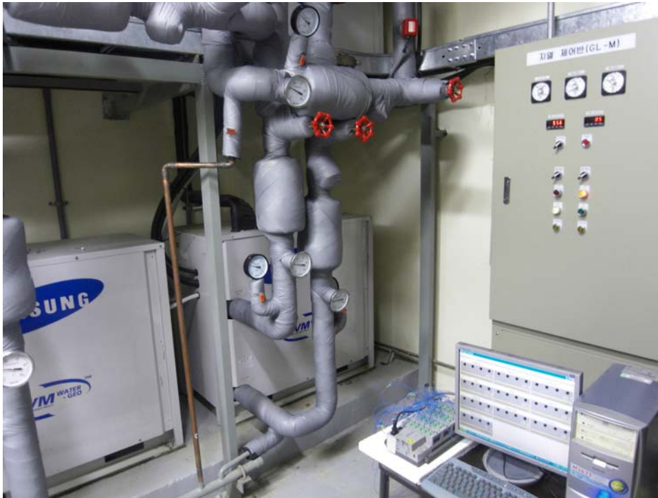
Photo. 2. Ground source heat pump outdoor unit
