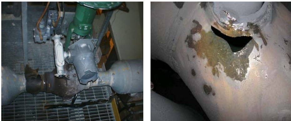
Fig. 3-4 Pipe of damage example
