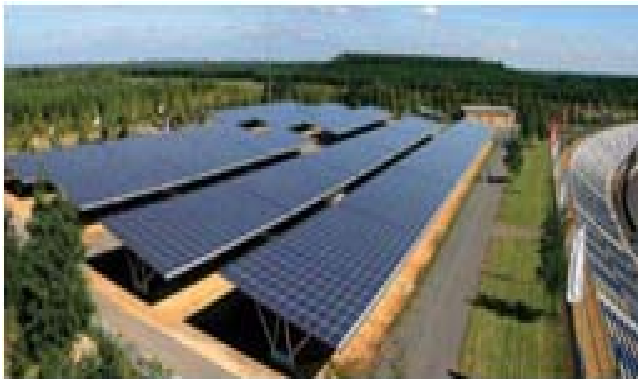
Fig. 3-1 Slope fixed PV array
