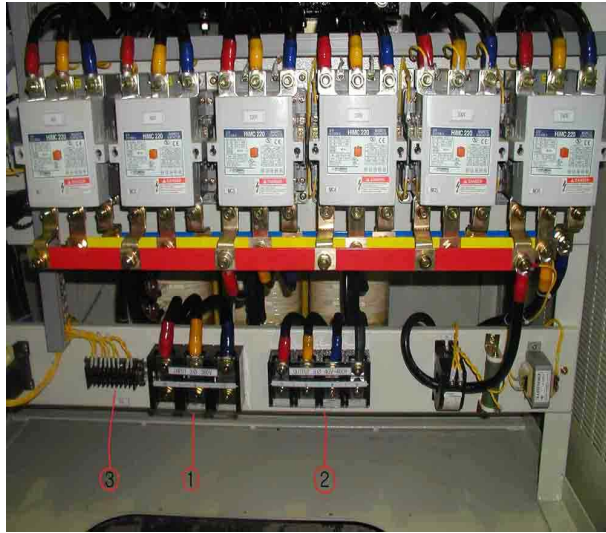
(a) The Inside Circuit Picture
