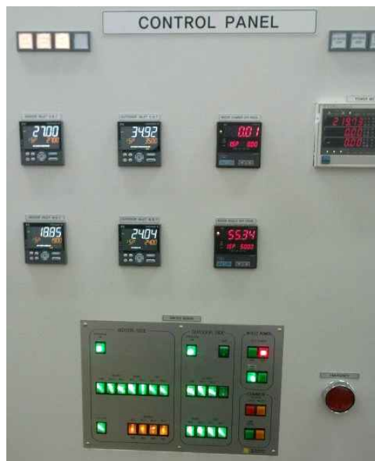
Fig. 2.4 Control panel of psychrometric chamber.
