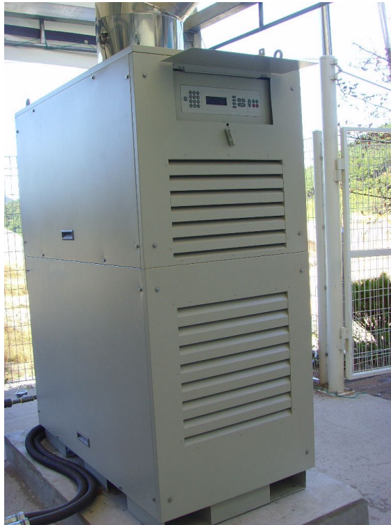
Figure 6. Micro Gas Turbine ( MGT C30, Capstone社 America)
