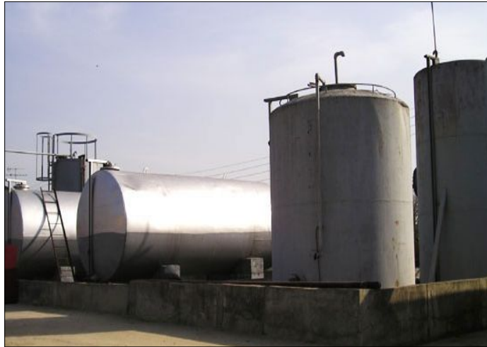
Fig. 4.48. Photograph of tanks for storing oil.
