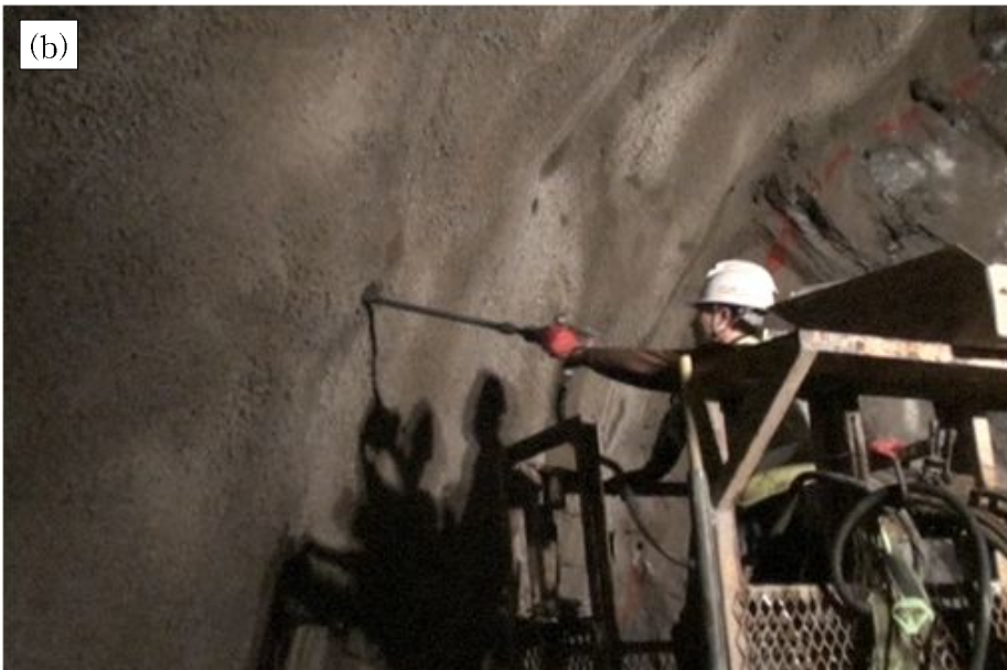
Figure 6.6 Installation process of rock and spiral bolts in a borehole: (a) Injection of resin, (b) insertion of supports, (c) completion of installation, (d) pull-out test and data acquisition.
