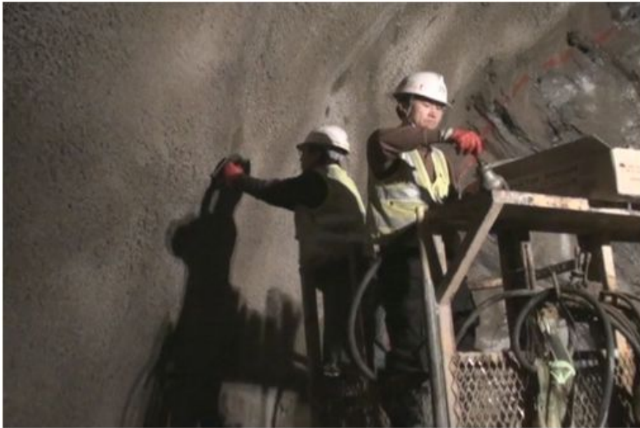
Figure 6.5 Installation of rock bolts and spiral bolts for pullout tests in a tunnel.
