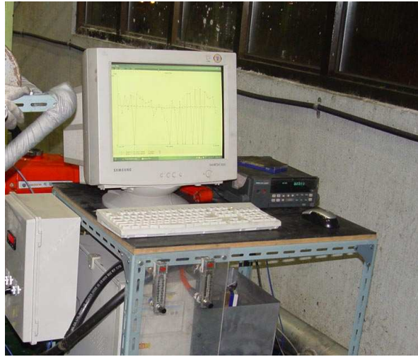
Monitoring system of measurement temperature
