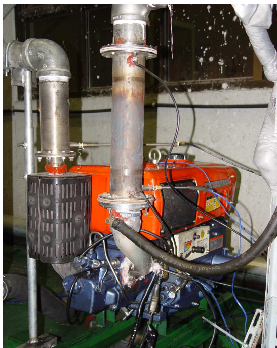
(a) Photography of preheater heater
