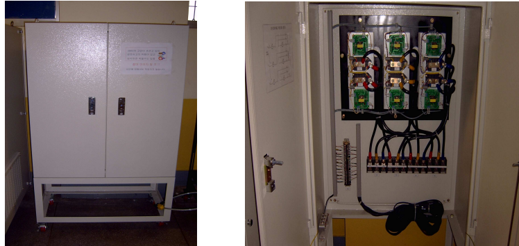
Fig. 19. The switch panel for various fault simulation
