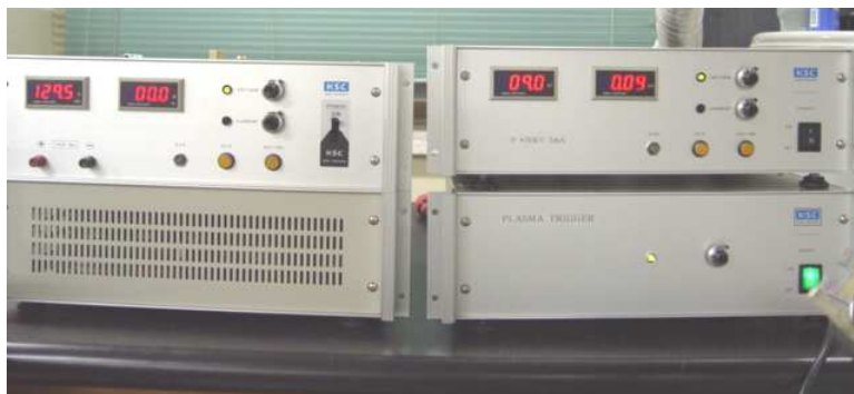
Fig. 3-4. Photograph of a power supply system.
