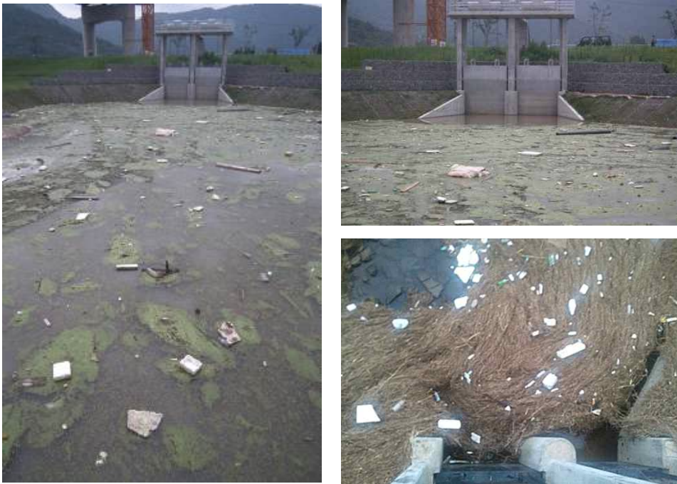
Fig. 3-39 Photo of contaminants flowing into the water gate during rainfall
