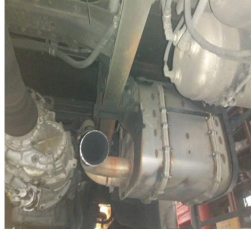
(b) Large exhaust pipe
