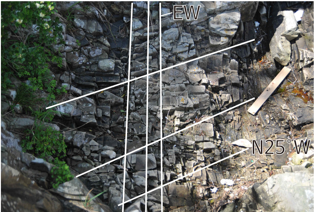
Fig. 28. Structural joint developed at the edge of Anjang-seom(island).
