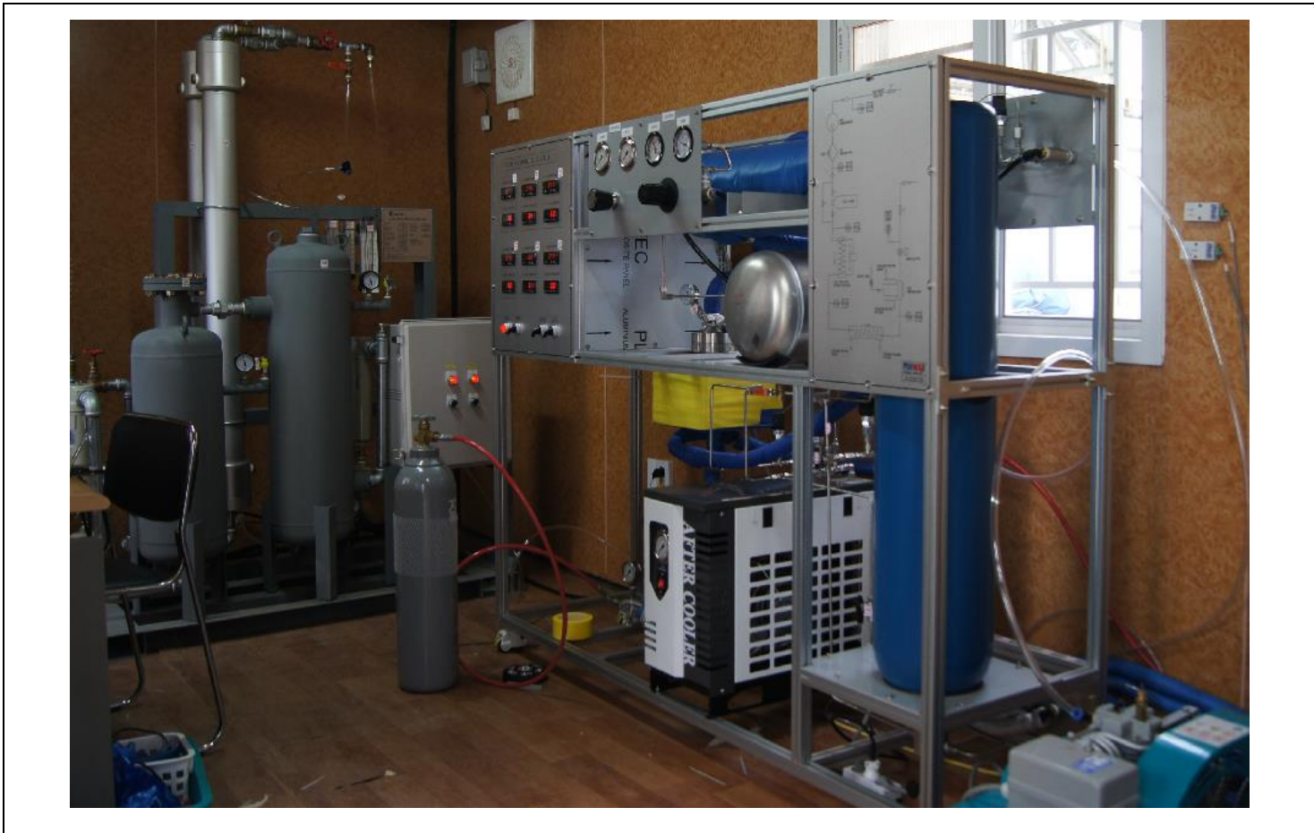
Figure 3.10 Photograph for CO 2 liquefaction equipment
