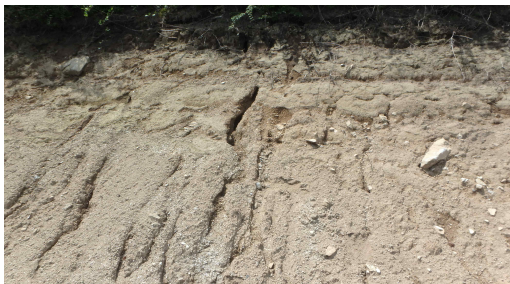
(a) Piping 현황
