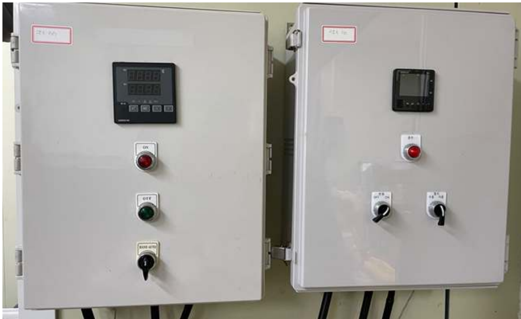
Fig. 2.9 Image of heating controller
