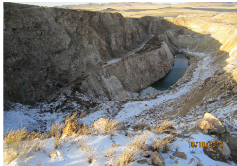
Failure of tailing dam
