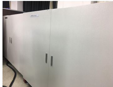
(b) Exterior of battery bank
