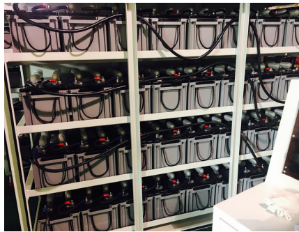
(a) Interior of battery bank
