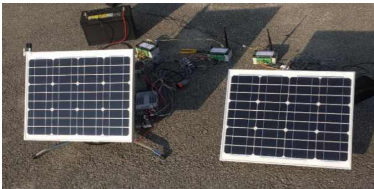
Fig. 23. On a cloudy day fixed/tracking PV system measurement
