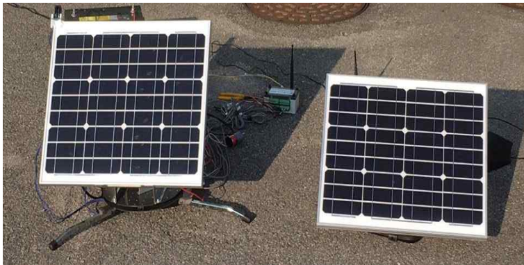
Fig. 22. On a clear day fixed/tracking PV system measurement
