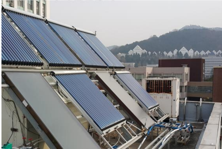
Fig. 3.1 Photograph of the solar collector
