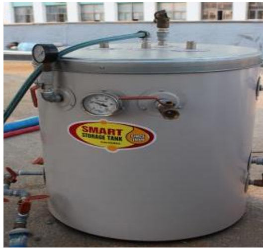
Fig. 3.6 Photograph of the storage tank
