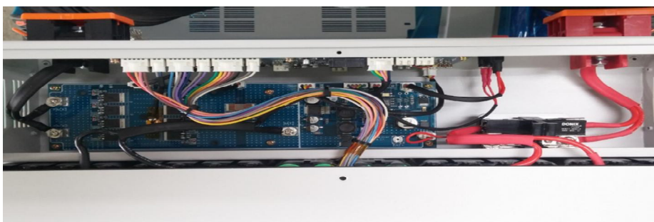
Fig. 4-60. PCM and BMS in the energy storage system(SP48M)
