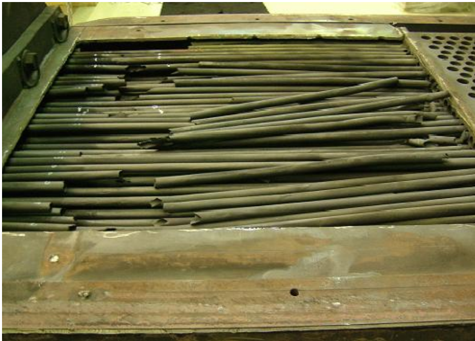
Fig. 1 -2 Damaged MSR tubes
