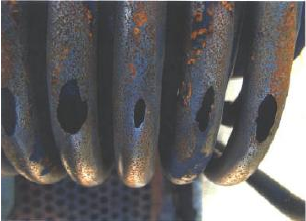
Fig. 1-3 Erosion in the MSR U-bend
