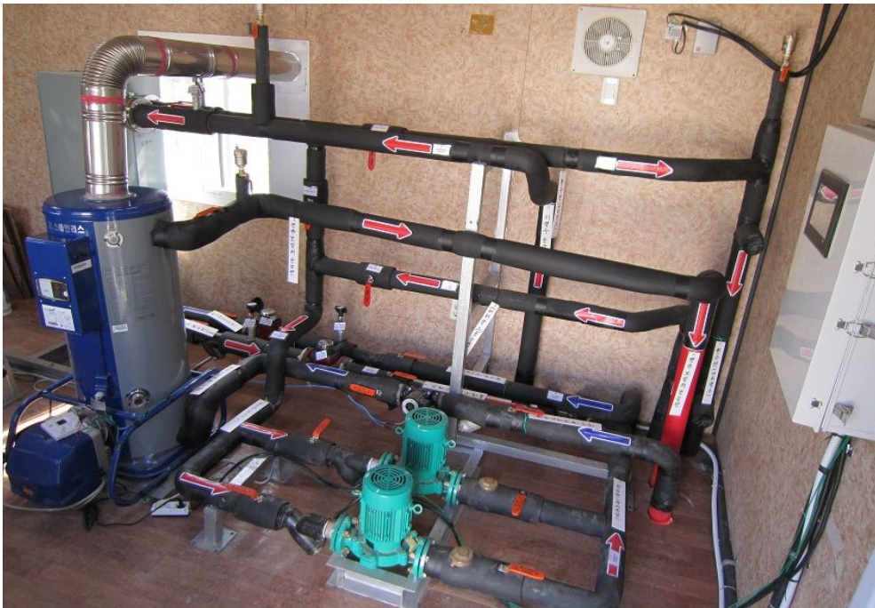
Fig. 4-5 Deep-geothermal system equipment of naju-site
