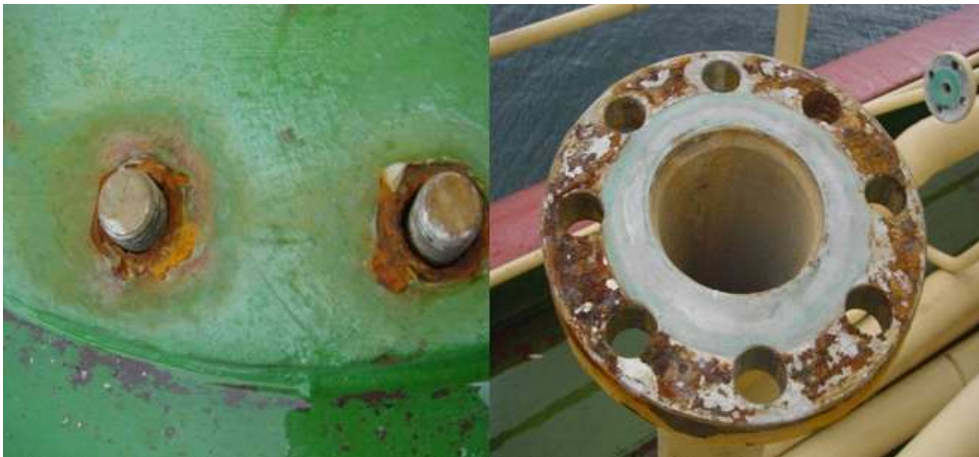
Fig. 2.3 Crevice corrosion: (a) Mechanism, (b) crevice corrosion at plant connection.
