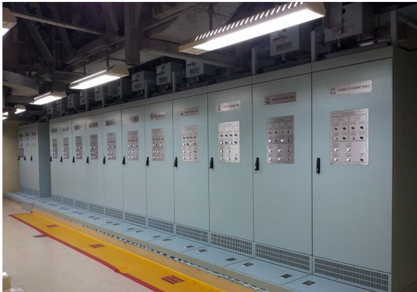
Figure 7. CEDMCS digital control panel
