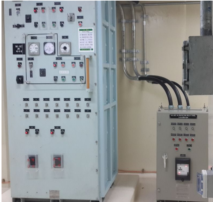
Figure 38. MG Set control panel and new protection panel
