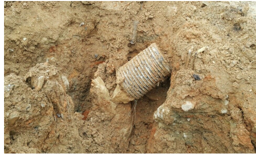
Figure 4.32 Destruction of C.P.R bulb
