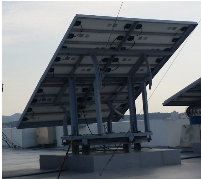
Fig. 9 The photo of semi-fixed array
