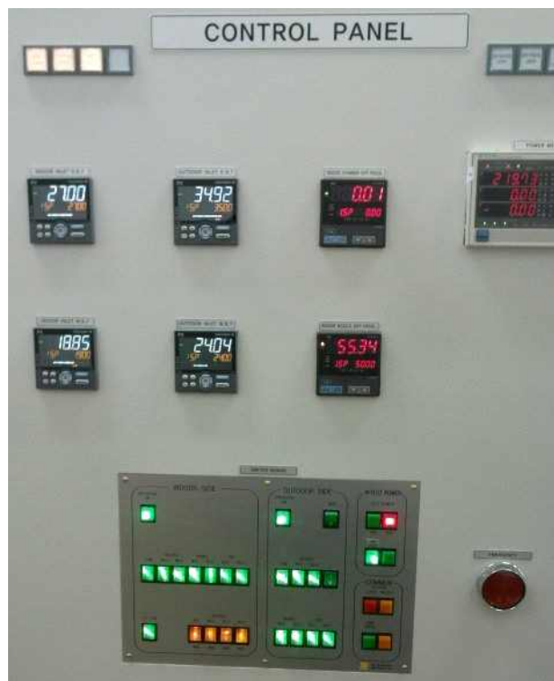
Fig. 2.4 Control panel of psychrometric chamber.
